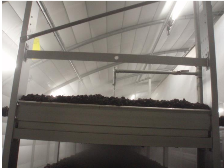
Fig. 4 Overhead sprinkler irrigation system
